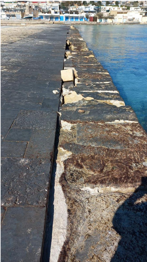
Photo 4: 24/02/2026 – General damage across sea wall
