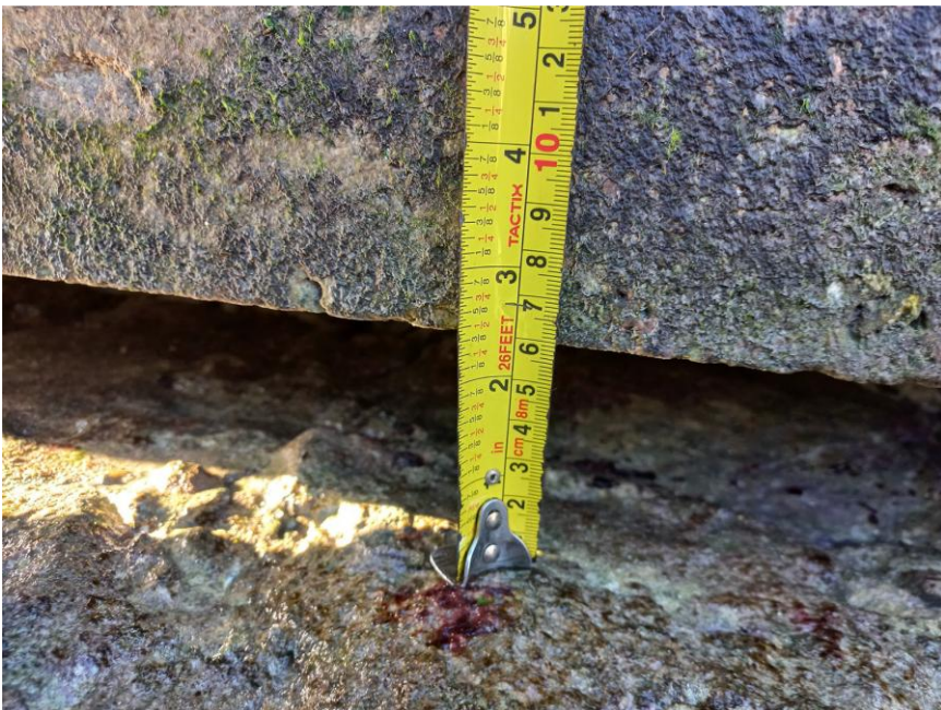
Photo 14: 24/02/2026 – Underlying sand and/or fill material washed out resulting in the formation of voids
