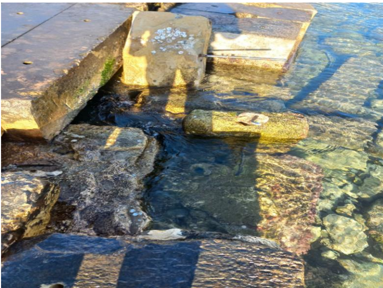
Photo 9: 24/02/2026 – Severely damaged lintels spanning over the canal
