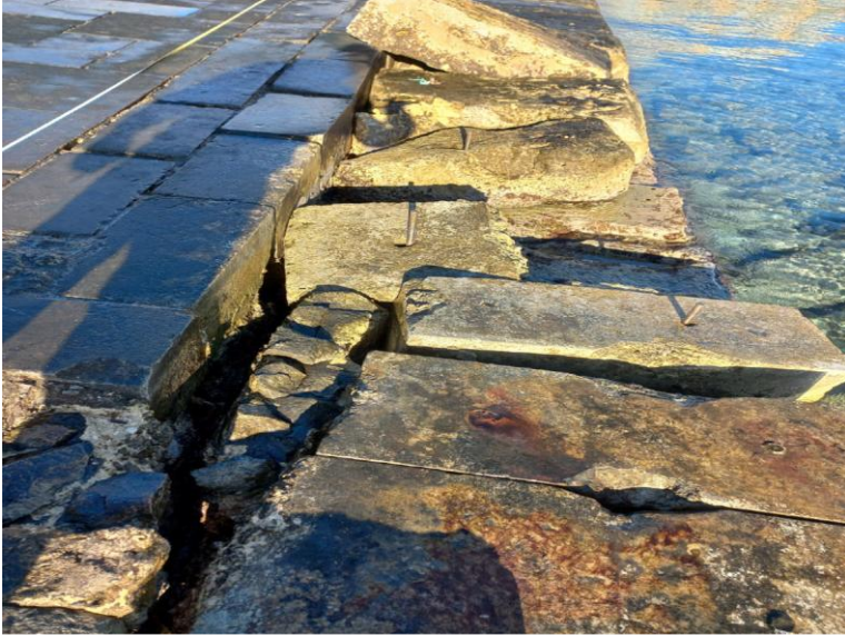
Photo 10: 24/02/2026 – Displacement of the outer limestone masonry blocks and the failed dowels
