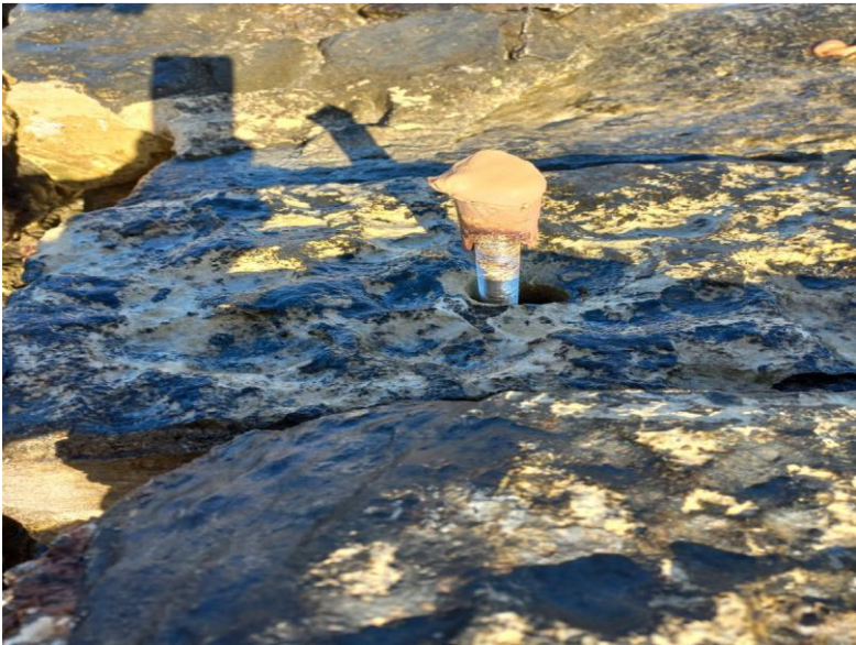
Photo 11: 24/02/2026 – Bearing failure of the dowels
