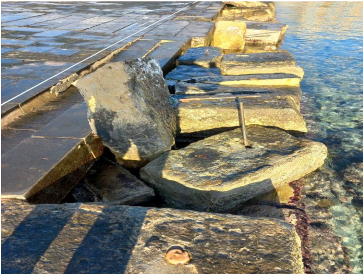
Photo 7: 24/02/2026 – Displacement of the outer limestone masonry blocks and the failed dowels
