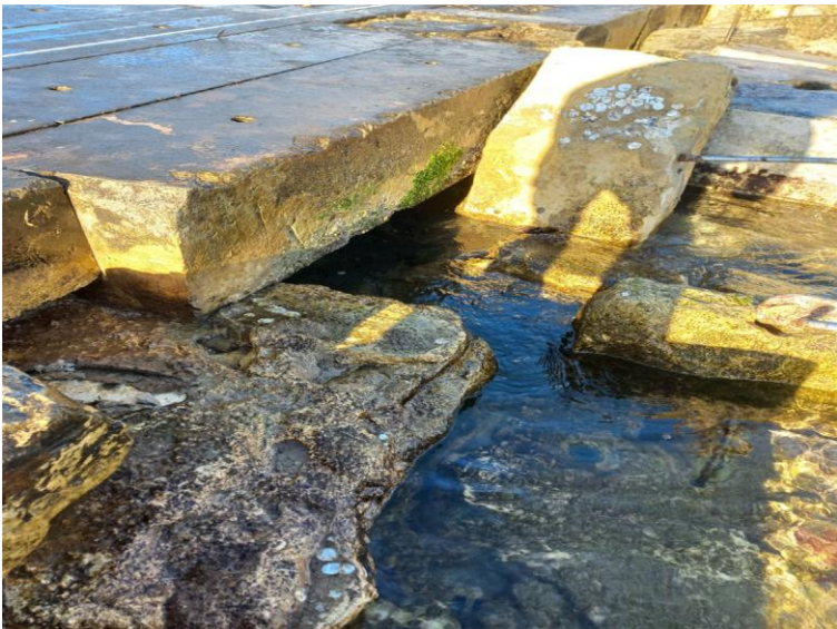
Photo 8: 24/02/2026 – Severely damaged lintels spanning over the canal
