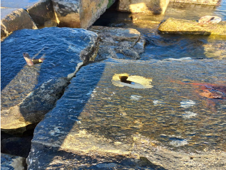
Photo 13: 24/02/2026 – Bearing failure of the dowels and subsequent contact interface
