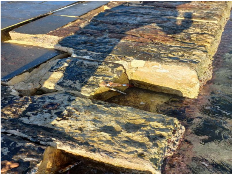
Photo 12: 24/02/2026 – Bearing failure of the dowels
