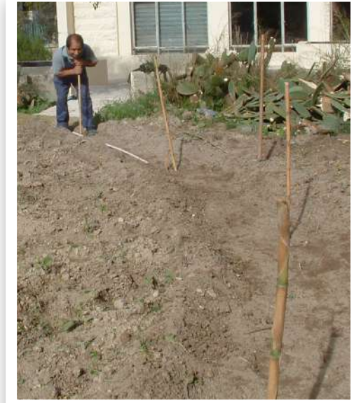
The nature trail was the first phase of the project, here already dug and marked out in preparation for the aggregate layer
