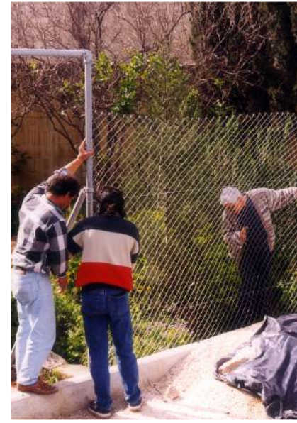
Installing a wire fence along the main border to reduce damage from errant balls
