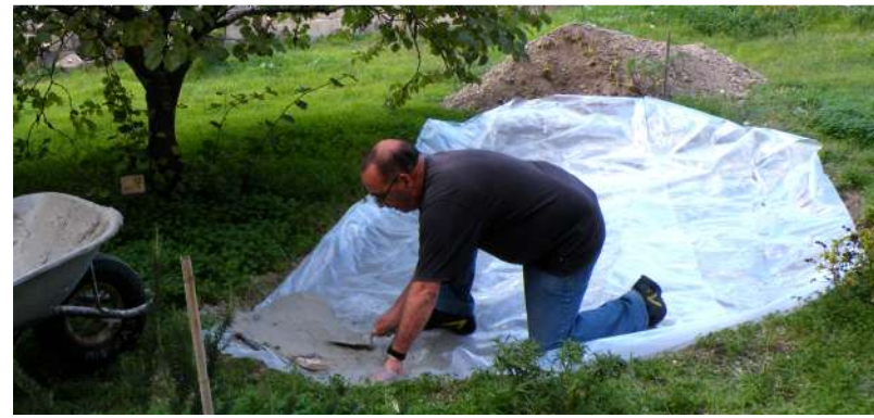
Construction of the freshwater pond under way - apart from polythene liner this pond was also given a cement base
